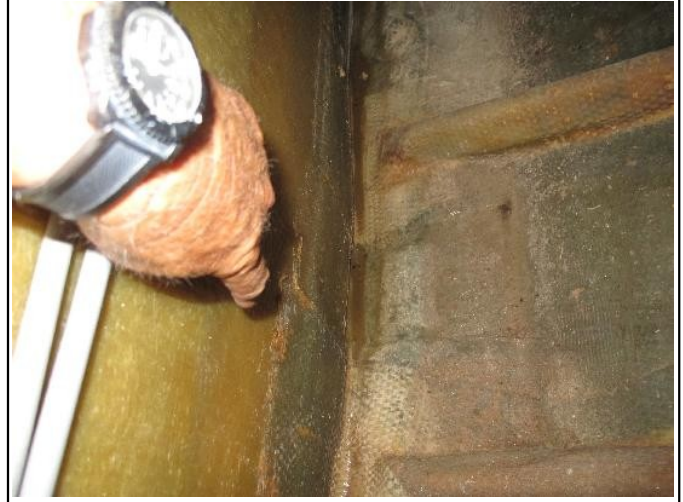
Fiberglass repair tacky at stringer under port stateroom floor
